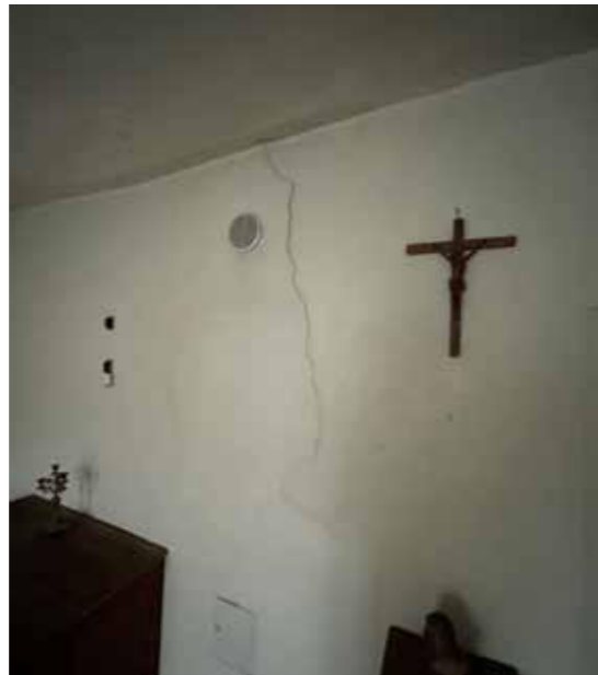
Fissure mur refend R+1
